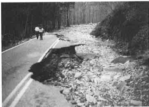
Flooding in Rockbridge Co.
