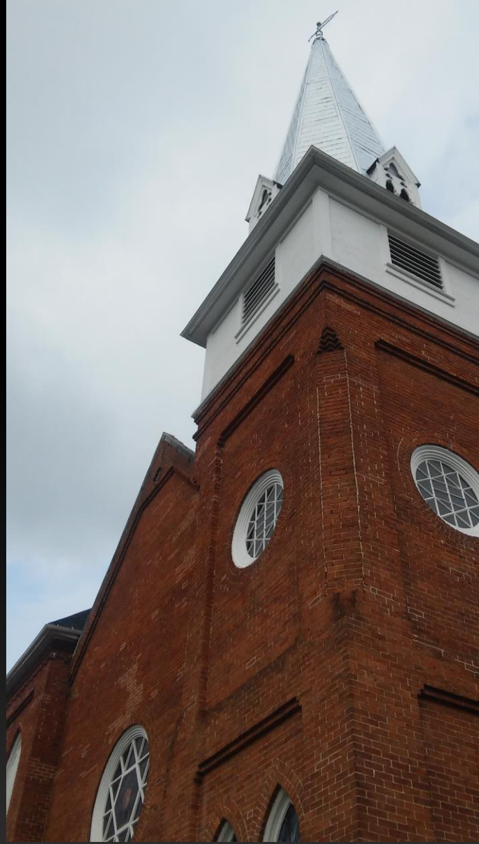
First Baptist Church, N. Main Street -- 2015 After Steeple Renovation (supported by HLF and City of Lexington)
