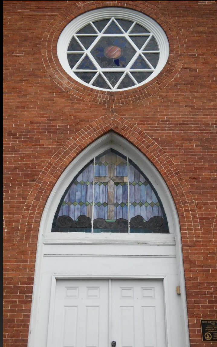
First Baptist Church, N. Main Street -- 2015 After Steeple Renovation (supported by HLF and City of Lexington)
